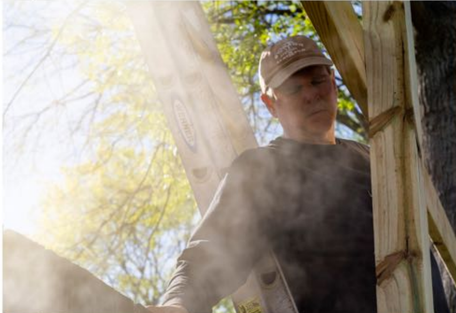
My father, Kimdell Lorei, takes a moment to rest while building a pergola in the backyard of our house.
