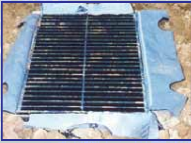
Installed Siltsack held in place by grate.
