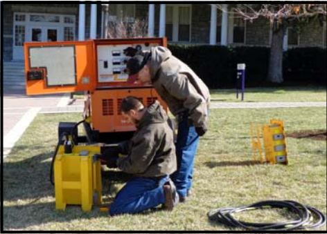
Electricians Mark Campbell and Chris Nazelrod check the generators on the Quad
