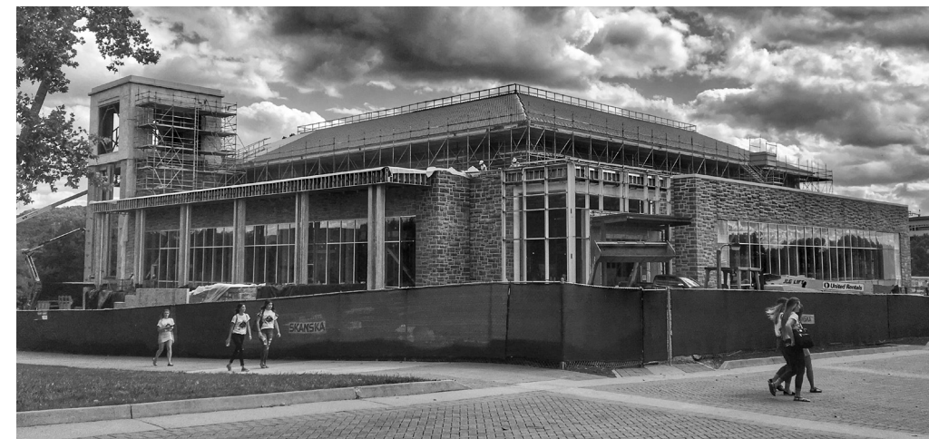
A new dining hall under construction in late summer 2017 on the footprint of Gibbons. (Courtesy Frank Doherty)
